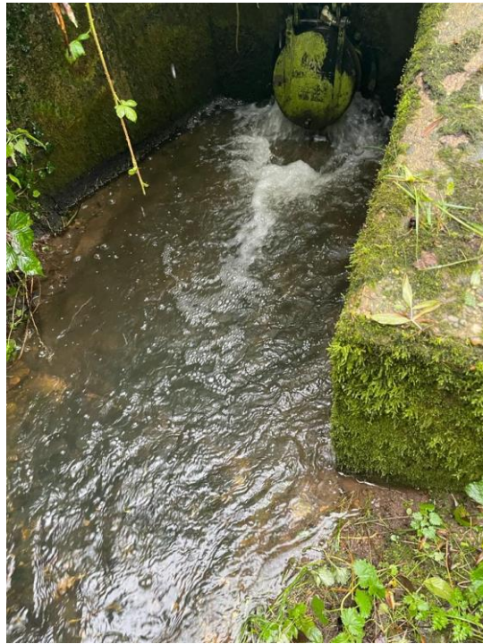
Flood Attenuation Area – Lady Franklin Drive Friday 19 th October 2023 Showing Dry storage Area and unattenuated discharge.
